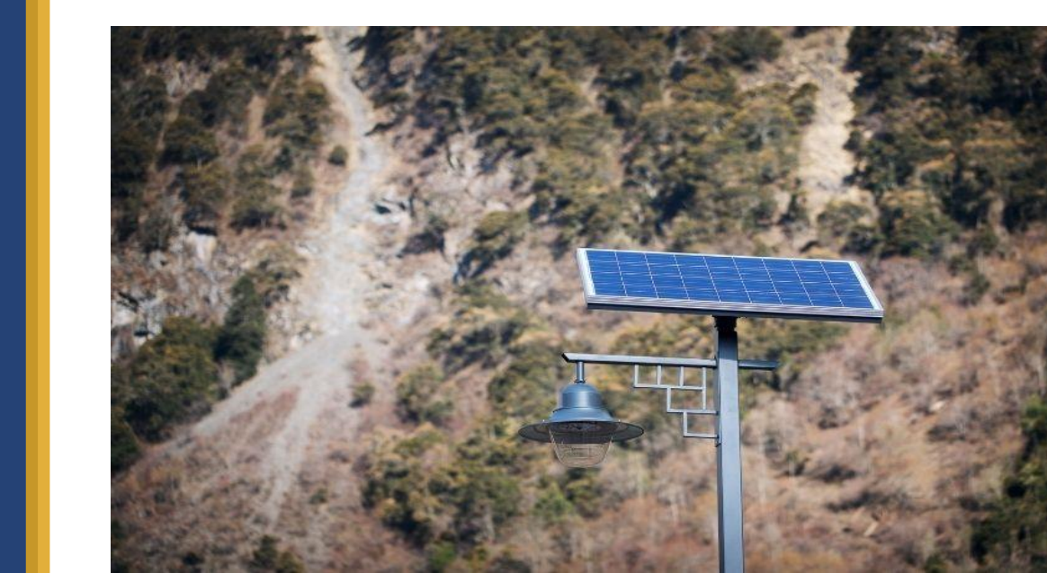
Figure 15. Solar outdoor lighting
